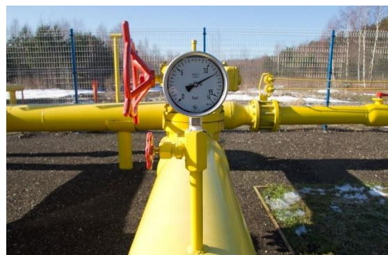
(Photo: Natural gas distribution; source: www.delfi.ee )
