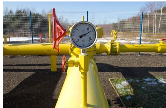
(Photo: Natural gas distribution; source: www.delfi.ee )
